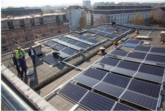
Figure 41: DREWAG photovoltaic system
