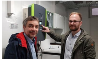
Figure 40: Released press photo shows our project managers in the utility room of the DFH
