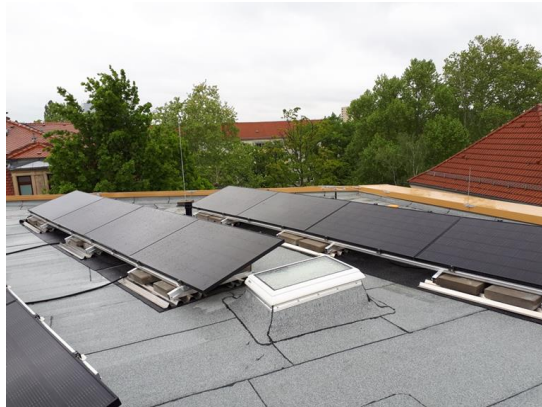
Figure 54: Photovoltaic system on the District Future House
