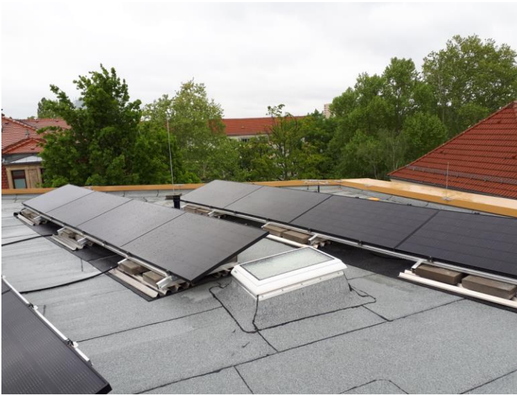
Figure 29: Photovoltaic system on the future house
